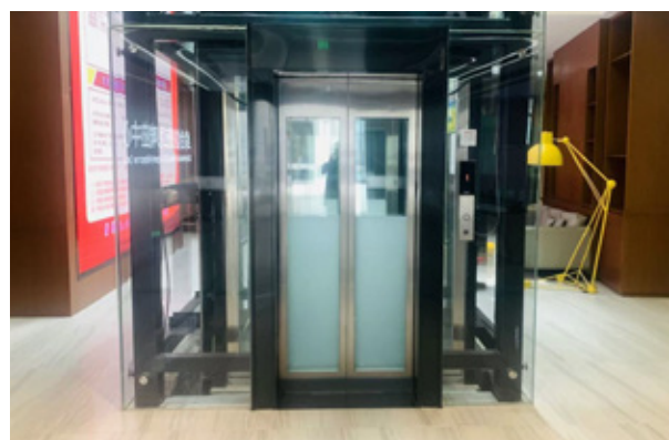
The elevator outside the Command Center
